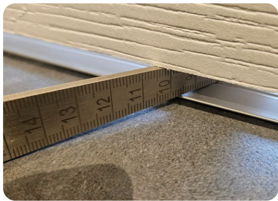
Door undercuts corrected to 10 mm
